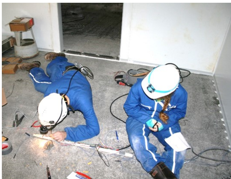
Installation of the ultrasonic passive and active sensors inside the salt rock mass under the experimental cooling chamber
